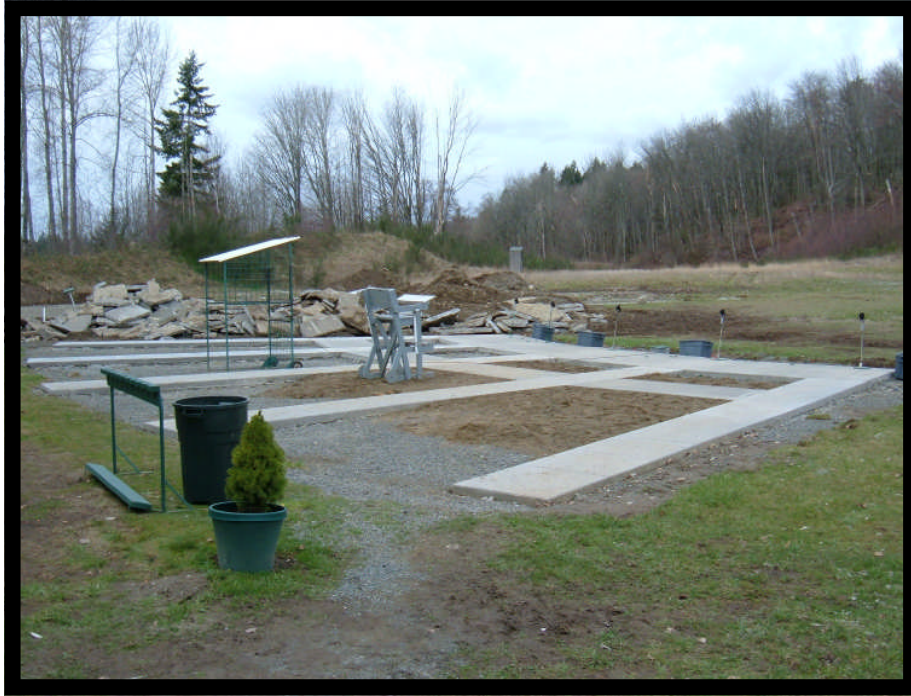
Trap #1 new cement field with wheelchair wide walkways and a connecting path. Notice the pile of cement from the old walkways.
